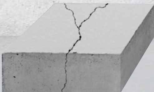
Random cracking is amongst the most costly and aggravating problems facing concrete contractors.
